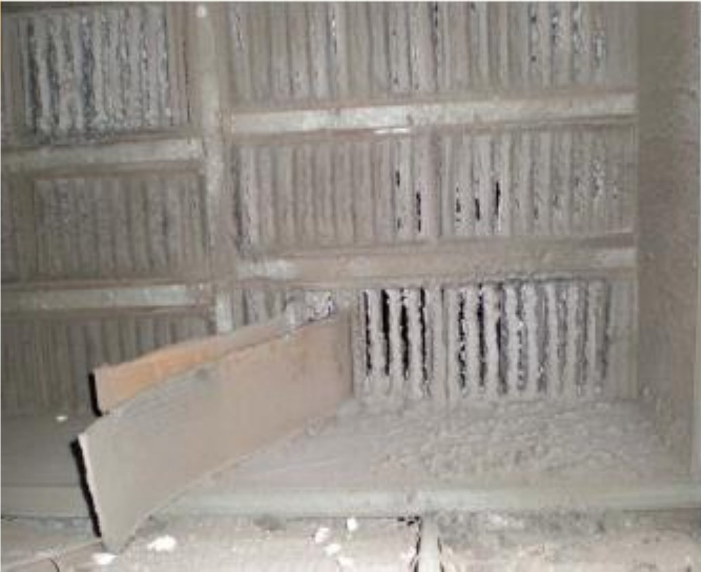
Air Silencer at Festival Theatre return air ductwork caked with dust
